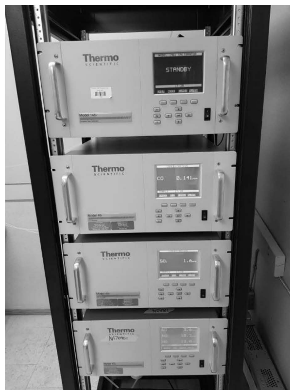
Example of Site C gas monitors
